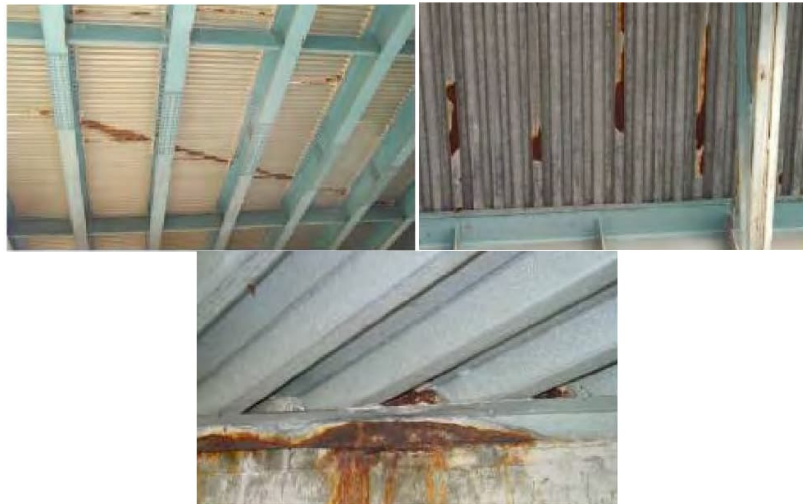
Figure 1, clockwise from upper left: (a) Corrosion at concrete through-crack locations; (b) Corrosion at lower corrugation valleys; (c) Corrosion at connections. All images reproduced from MDOT report [2].
